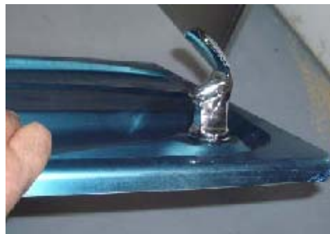
Exchange Bubbler hardware.
